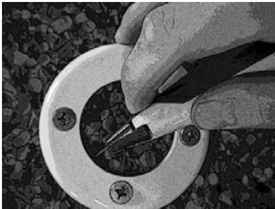
Trim liner from return opening.
